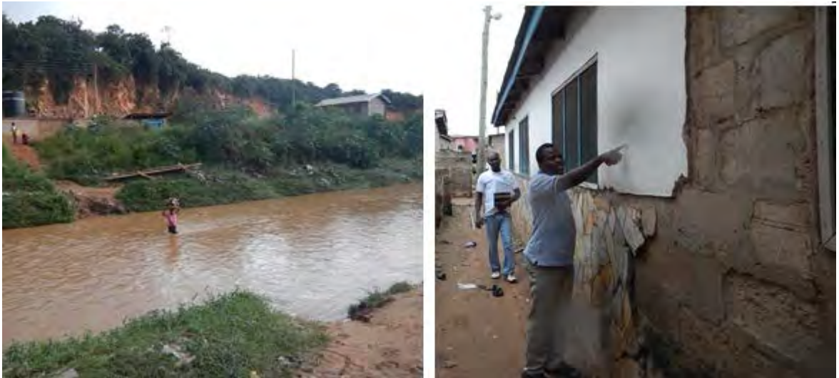
Figure 29: Alogboshie : washed out bridge (left), historical water level (right).
