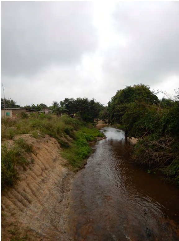
Figure 15. Downstream of bridge (stop 1) – on the left the river bank shows signs of erosion and sedimentation in the river bed. The houses build on the river bed are vulnerable to flooding.
