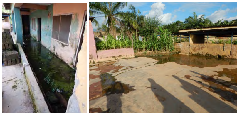
Figure 5. Asnoyeboa: abandoned school building (left) and ground water seeping through concrete court yard (right)
