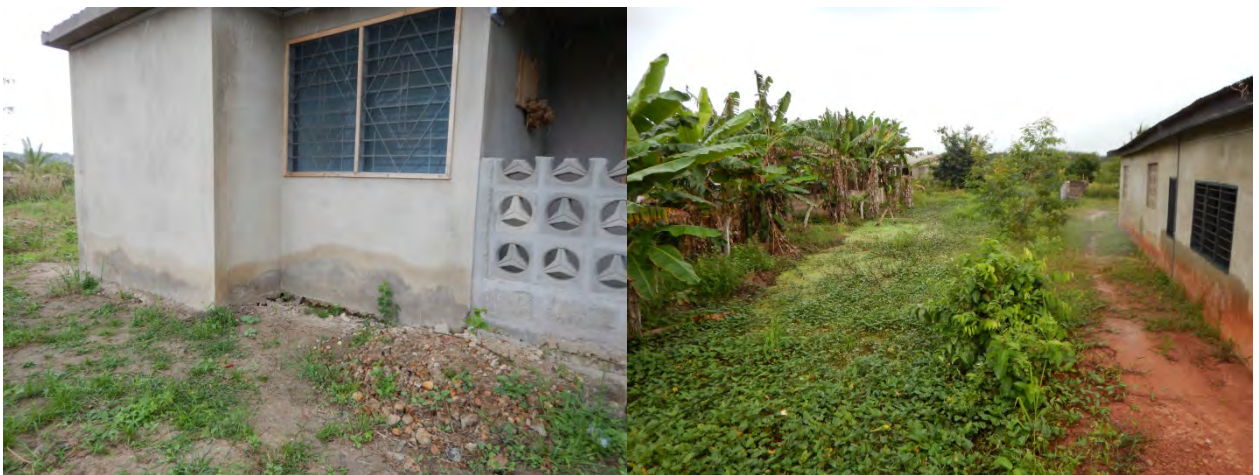
Figure 18. Houses within Kwapro community of which the foundation is affected by regular flooding.
