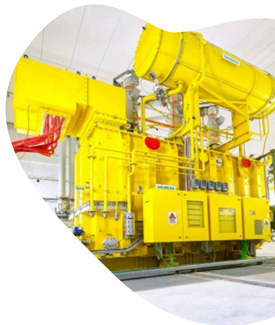
Arbarello HV-MV Primary Substation
