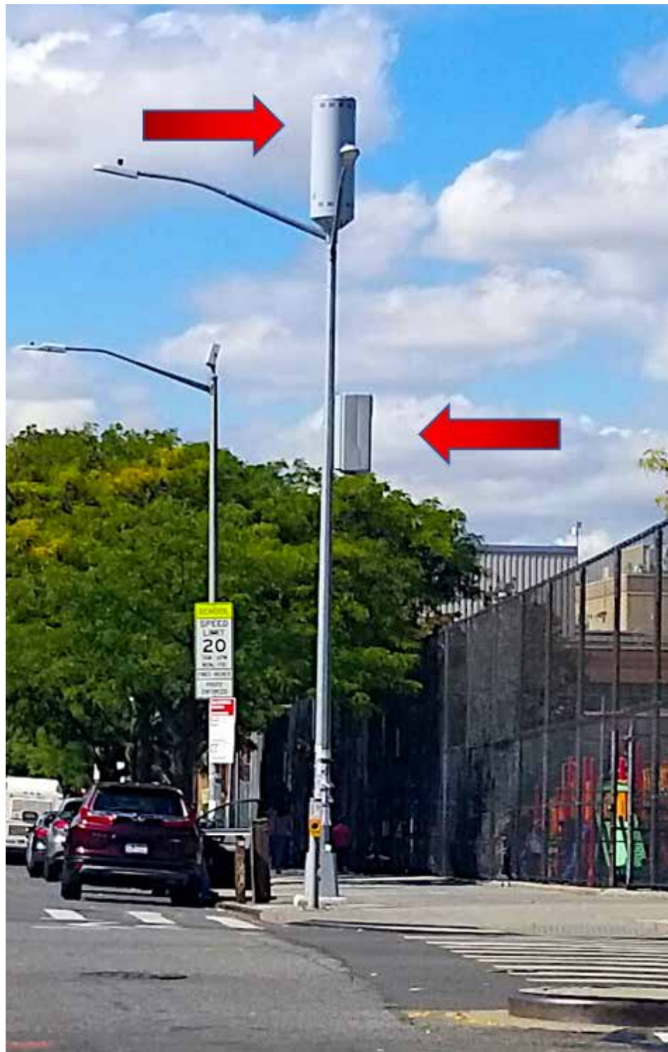
Pole-mounted 5G and small cell antennas at PS 506, corner of 4th Avenue & 60th Street, Brooklyn, NY. Photo credit: Les Jamieson
