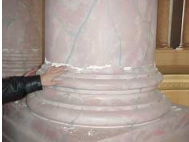
Figure 3.1.4 Cracking of Architectural Plaster at the Base of an Interior Masonry Buttress of the Legislative Building in Olympia.
