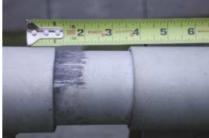
Figure 4.1.3 Slipping of Handrail on Holgate Bridge.
