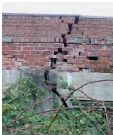
Figure 3.1.10 Shear Failure of a Perimeter Lintel of an Old Single-Story Masonry Warehouse in Kent.
