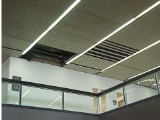
Figure 5.1.2 Partial Failure of a Metal Suspended Ceiling at Sea-Tac Airport.
