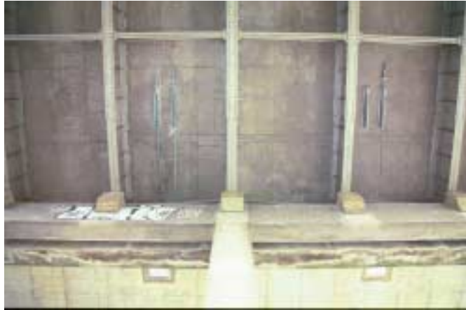
Figure 4.2.6 Damage to Restrainers.
