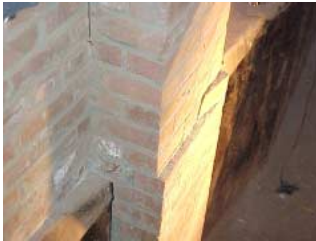
Figure 3.1.3 Differential Movement between the Drum and Lower Masonry Portion of the Legislative Building in Olympia.
