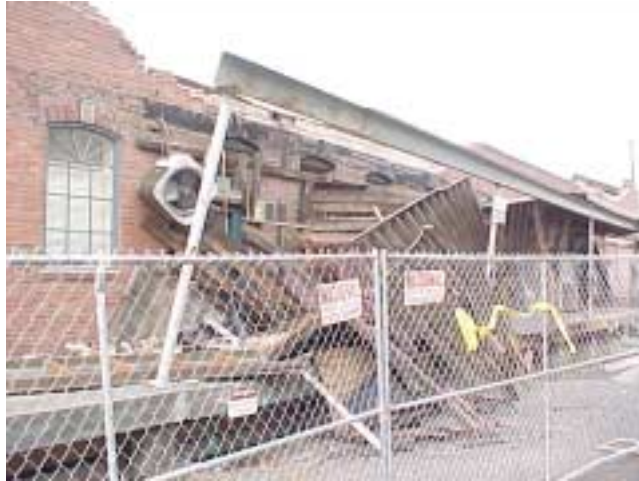
Figure 3.1.13 Partial Collapse of the South Façade and Failure of the Loading Dock Canopy of the Seattle Chocolate Factory in Seattle.
