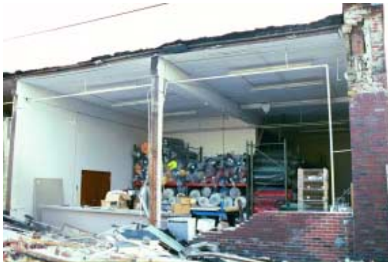
Figure 3.1.14 Complete Failure of an Unreinforced Brick Wall along the North Face of the Acme Tool and Specialty Building on First Avenue South in Seattle.
