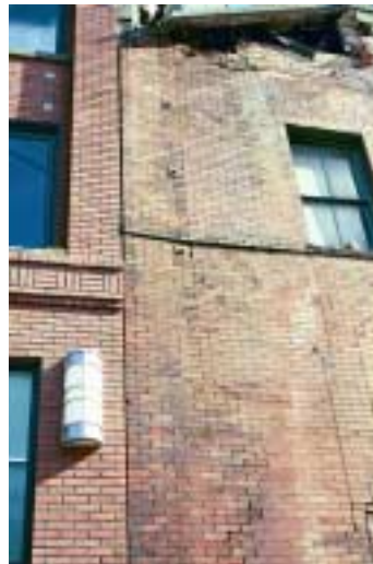
Figure 3.1.19 Brick Facade Forced Out-of-Plane by Pounding against an Adjacent Building in the 500 Block of First Avenue South in Seattle.
