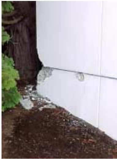
Figure 3.3.4 Damage in North Bottom Corners of Shear Walls of General Administration Building in Olympia.
