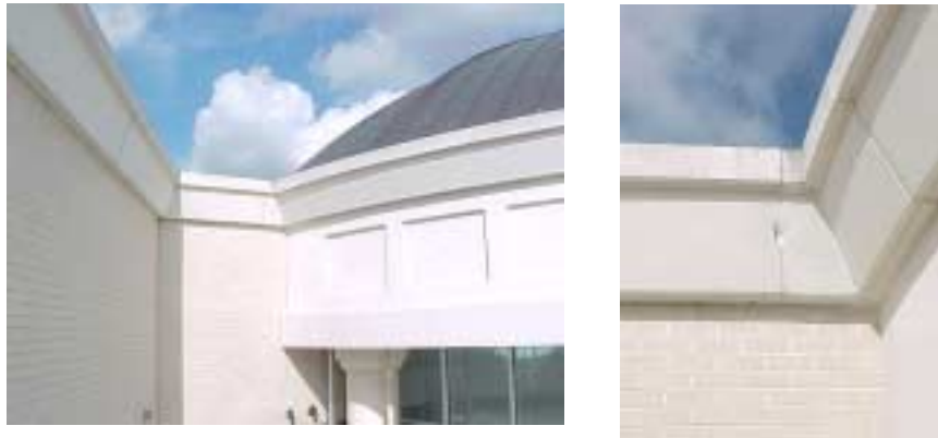
Figure 3.2.3 Evidence of Pounding at Kent Regional District Center.
