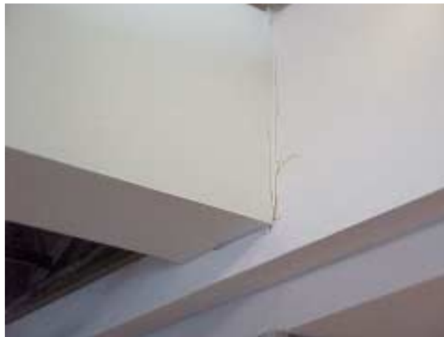
Figure 5.2.1 Cracking of Drywall Finish in a Beam-to-Wall Connection at SeaTac Airport.
