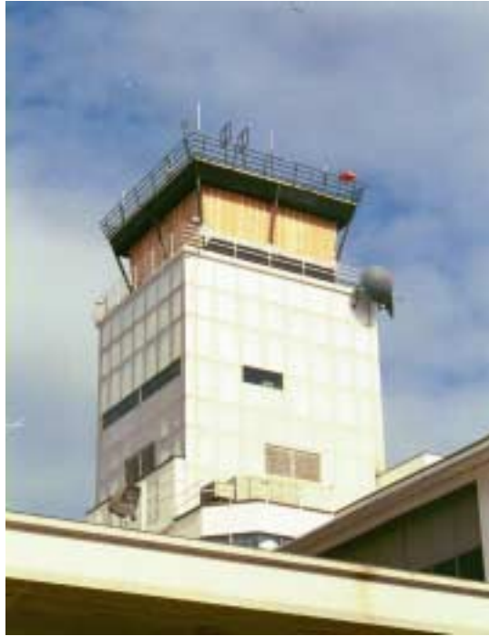
Figure 3.2.7 Damage to the Existing Sea-Tac Air Traffic Control Tower.
