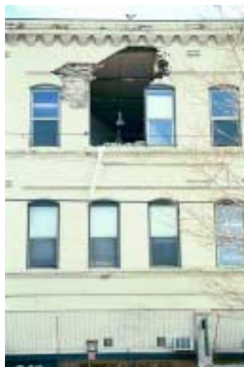
Figure 3.1.15 Out-of-Plane Failure of a Section of a Masonry Wall in a Three-Story Building in the 500 Block of First Avenue South in Seattle.
