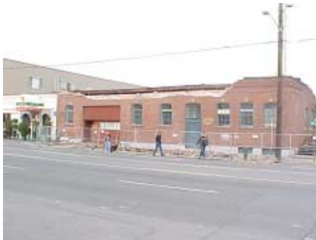
Figure 3.1.12 Collapse of the West Parapet of the Seattle Chocolate Factory in Seattle
