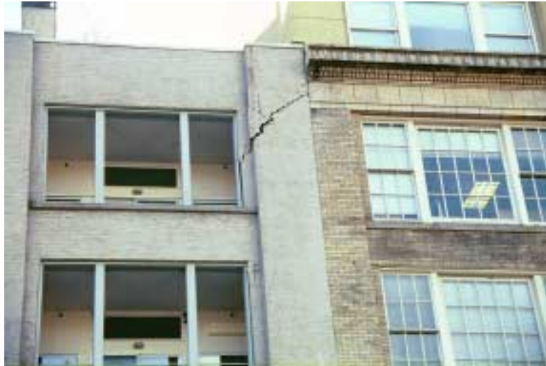
Figure 3.1.20 Localized Pounding Damage to a Brick Facade of a Four-Story Apartment Building at 515 Occidental Avenue in Seattle.
