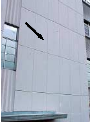
Figure 3.3.2 Diagonal Cracking in Central Shear Walls of General Administration Building in Olympia.
