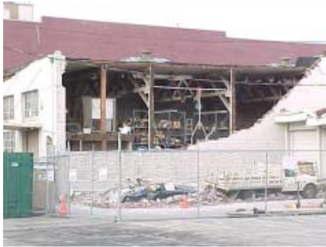
Figure 3.1.11 Failure of Masonry Facade of a Two-Story Wood Building in Seattle.
