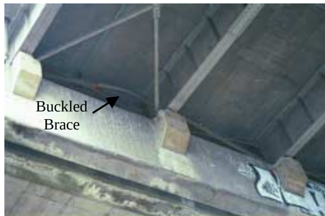
Figure 4.2.5 End Diaphragm with Buckled Braces in Bent 25.
