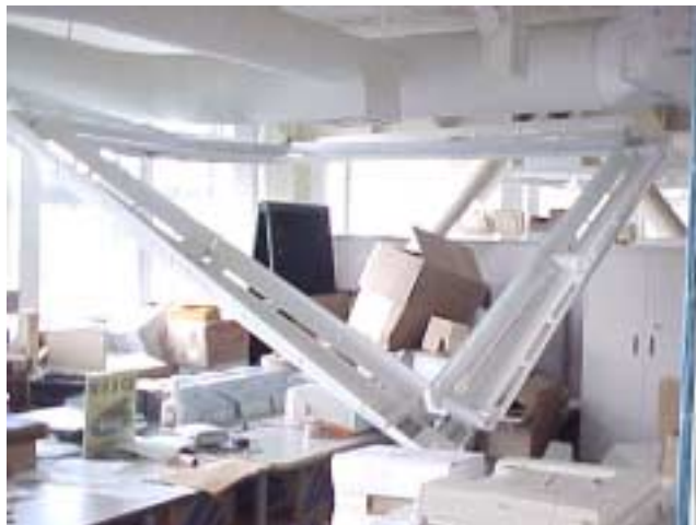
Figure 5.1.3 Failure of Suspended Lighting Fixtures in Starbucks Headquarters in Seattle.
