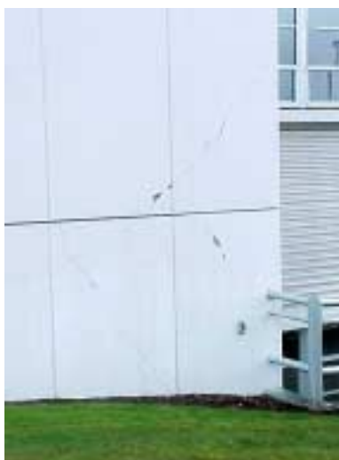
Figure 3.3.3 Diagonal Cracking in Corner Shear Walls of General Administration Building in Olympia.
