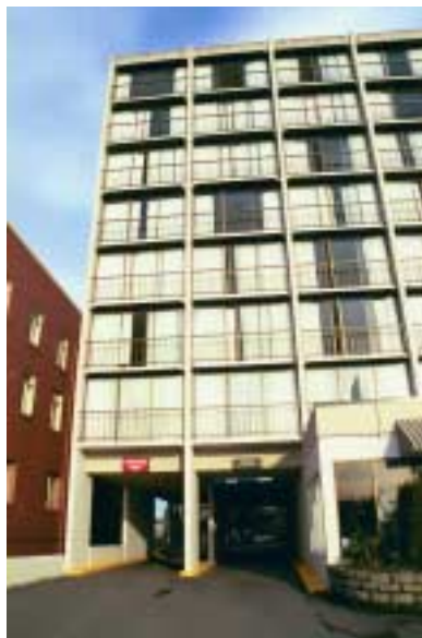
Figure 3.1.6 Section of the Ramada Inn in Olympia Showing Evidence of Differential Vertical Movement at Each Floor Level.
