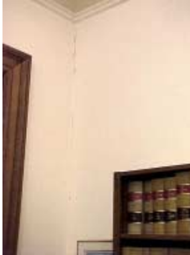
Figure 5.2.4 Vertical Cracking of Plastered Walls in the Supreme Court of the Temple of Justice in Olympia.
