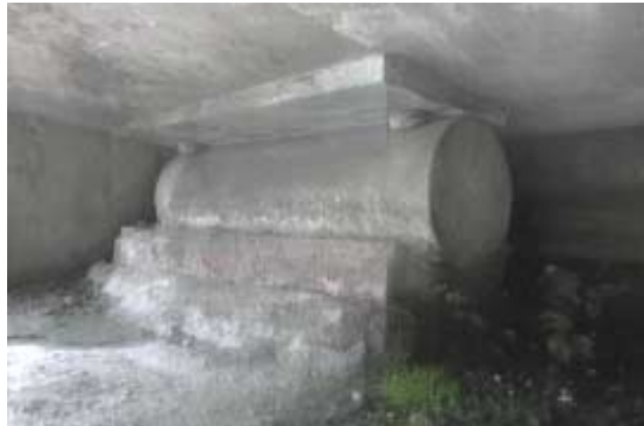
Figure 4.1.4 Displaced Roller on West End of Holgate Bridge.
