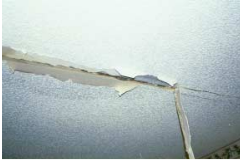
Figure 3.1.7 Differential Vertical Movement in the Floor Slab on the Eight Floor of the Ramada Inn.
