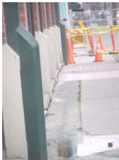
Figure 3.1.35 Separation between West Facade of the Cobalt Group Building in Seattle and the Sidewalk Showing Evidence of Rocking of the Building in East-West Direction.
