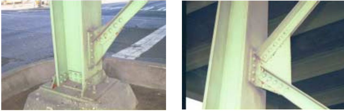
Figure 4.3.4 Paint Flaking at Column Base and Gusset Connections.
