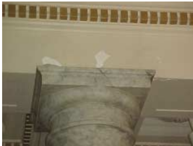
Figure 5.2.3 Spalling of Plaster in Legislative Building in Olympia.
