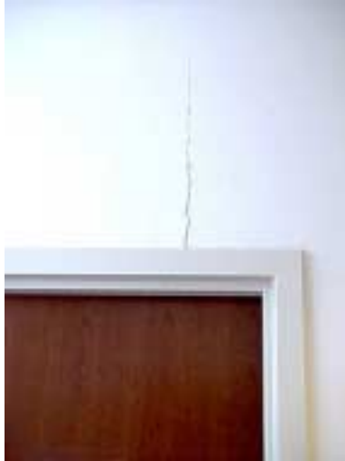
Figure 5.2.2 Vertical Cracking of Drywall Finish Above a Door Opening at Kent Regional District Center.
