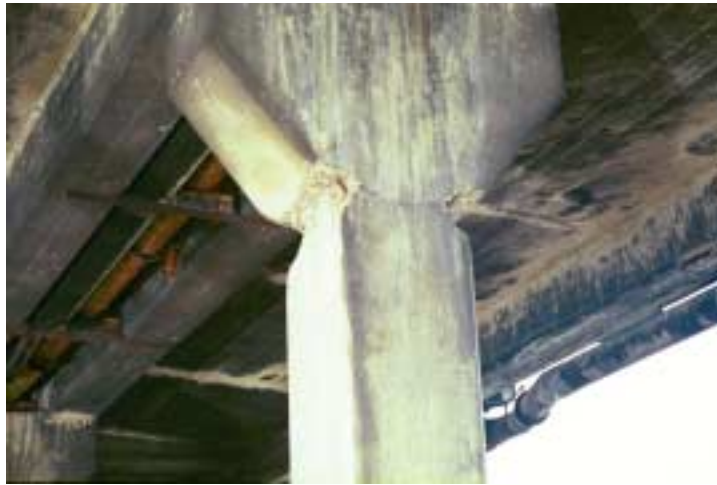
Figure 4.4.3 Concrete Spalling at the Base of Column Flare.
