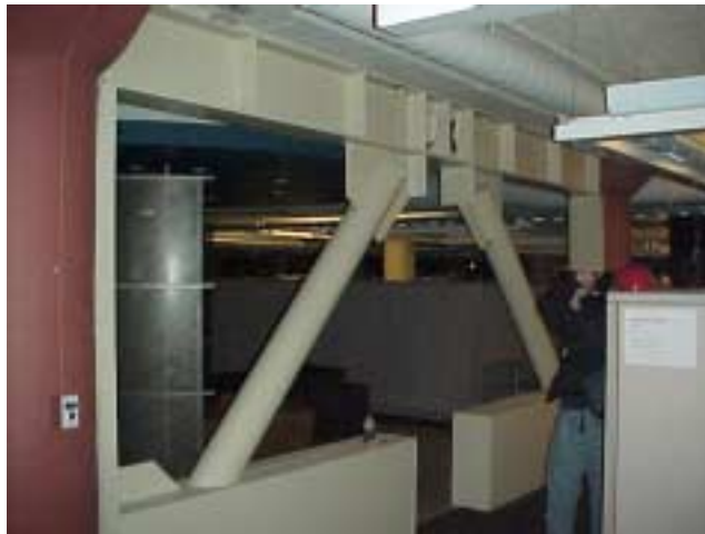
Figure 3.2.5 Chevron Eccentrically Braced Steel Frame Used to Seismically Upgrade the Starbucks Headquarter Building in Downtown Seattle.
