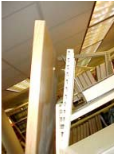
Figure 5.5.2 Failed Screwed Wood-to-Metal Connection at Top of a Leaning Bookshelf in the Main Library of the Temple of Justice Building in Olympia.
