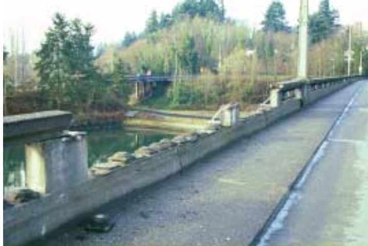
Figure 4.4.5 Failure of a Section of Pedestrian Handrail.
