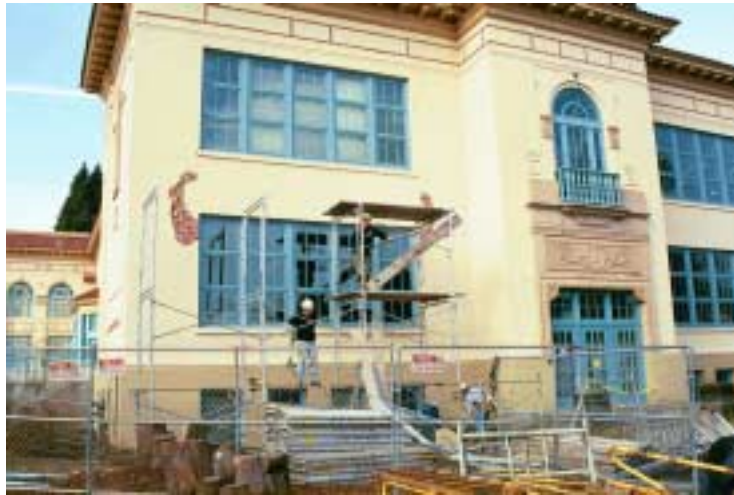
Figure 3.1.22 In-plane Cracking of Masonry Walls in the East Wing of Lincoln Elementary School in Olympia.
