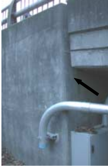
Figure 4.1.5 Cracked Abutment on East End of Holgate Bridge.
