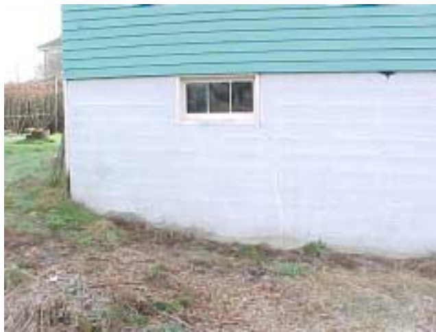
Figure 3.1.29 Cracking of the Concrete Foundation Wall of a Wood Frame House in Olympia.
