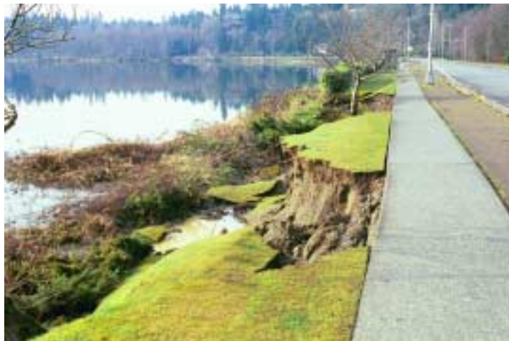
Figure 4.4.6 Soil Failure along the Shore of Capitol Lake.
