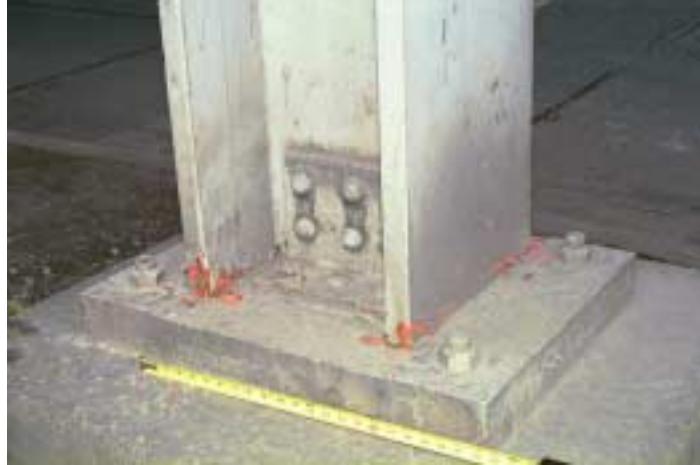
Figure 4.2.8 Yielding at Exterior Column Base of Bent 26.
