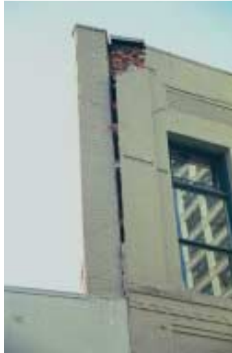
Figure 3.1.17 Permanent Gap between Perpendicular Walls in a Masonry Building along the 400 Block of Second Avenue of Seattle.
