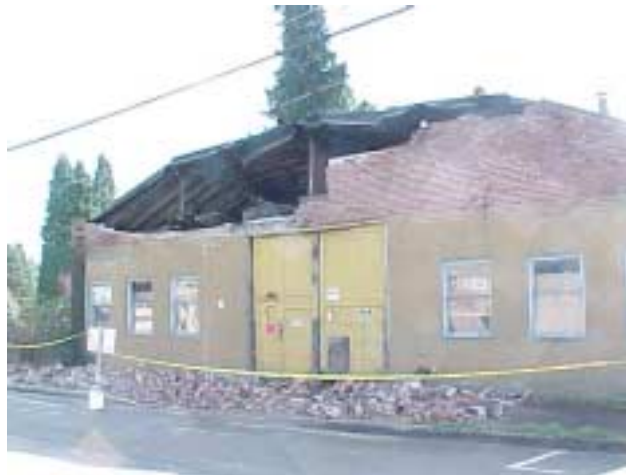
Figure 3.1.9 Out-of-Plane Failure of an Old Single-Story Masonry Warehouse in Kent.
