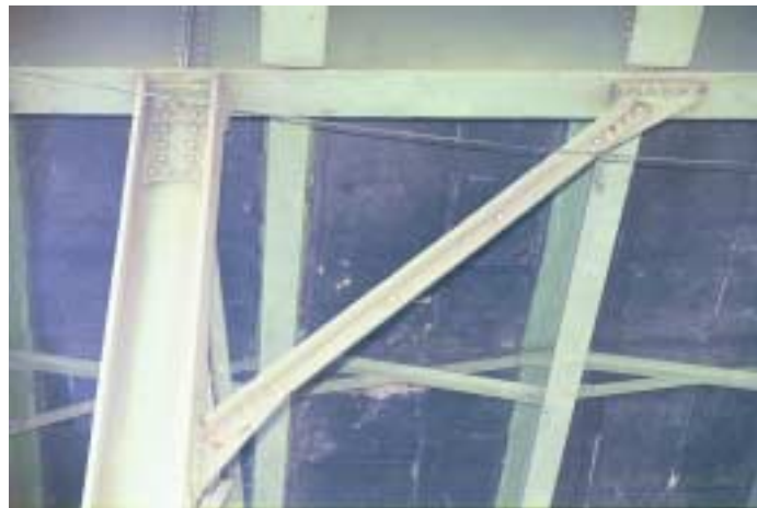
Figure 4.3.5 Paint Flaking at Knee Brace.
