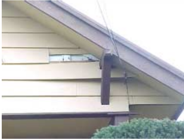
Figure 5.3.2 Damage to the Siding Boards on a Wood Frame House in Olympia.
