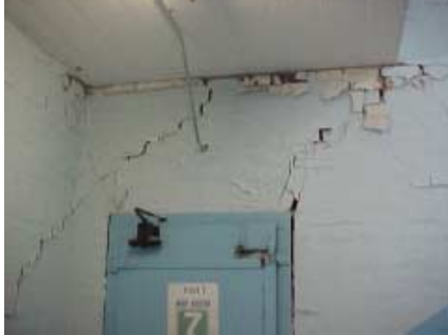
Figure 5.2.6 Severe Cracking of Masonry Stairwells in Starbucks Headquarters in Seattle.
