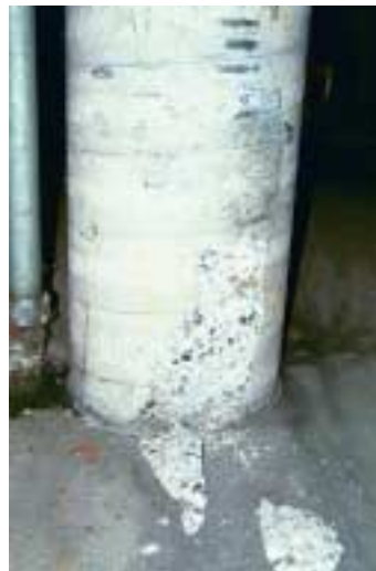
Figure 3.1.8 Spalling of a Reinforced Concrete Column in the Parking Structure Under the Ramada Inn.
