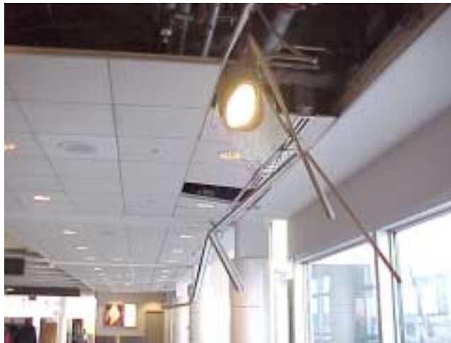
Figure 5.1.1 Partial Failure of a Suspended Ceiling at Sea-Tac Airport.
