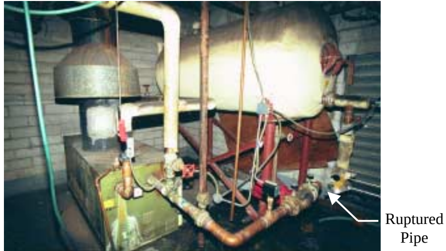
Figure 5.6.1 Rupture of the Supply Water Line to a 3000 Liter Storage Tank in the Roof Top Mechanical Room of the Ramada Inn in Olympia.
