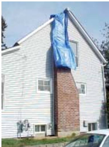
Figure 3.1.27 Chimney Failure in a Two-Story Wood Frame House in Olympia.
