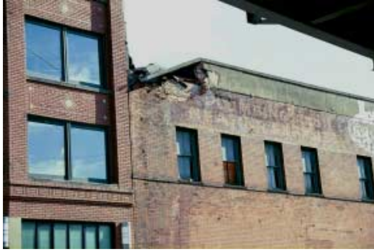
Figure 3.1.18 Partial Roof Failure Resulting from Pounding of Adjacent Building in the 500 Block of First Avenue South in Seattle.
