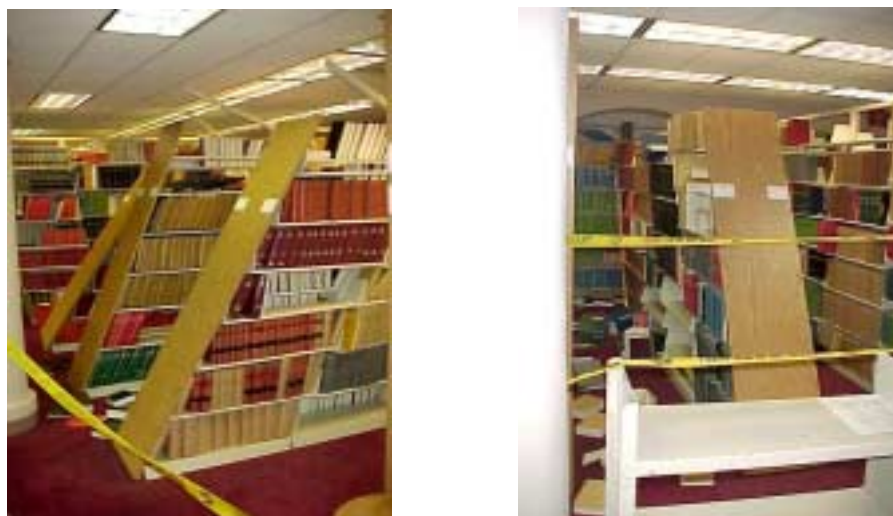
Figure 5.5.1 Failed Bookshelves in the Main Library of the Temple of Justice Building in Olympia.
