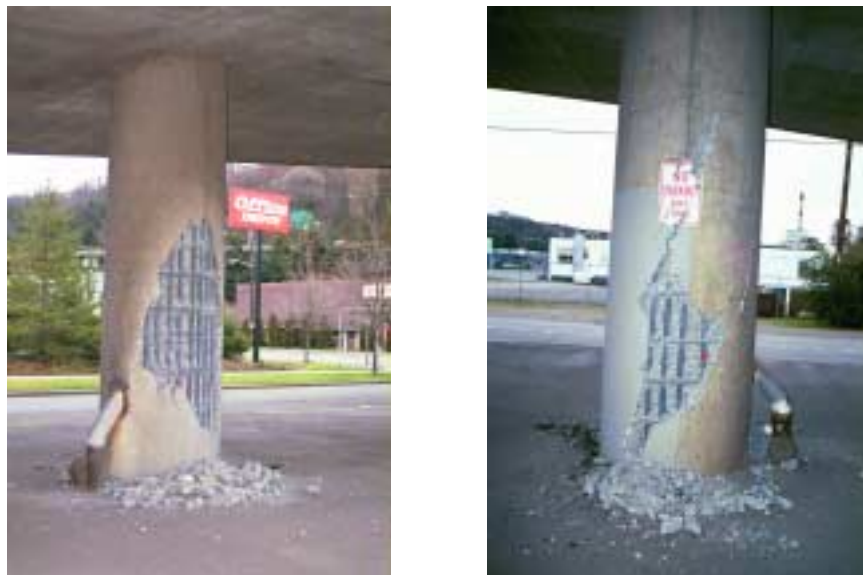
Figure 4.1.2 Cracking and Spalling of Concrete in Holgate Bridge Column.
