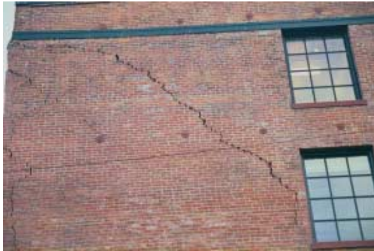
Figure 3.1.34 In-plane Cracking of the North Masonry Wall of the Cobalt Group Building in Seattle.
