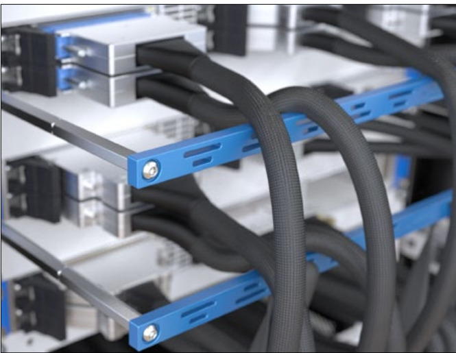
Rack Utilizing Cable Support Management Kits
