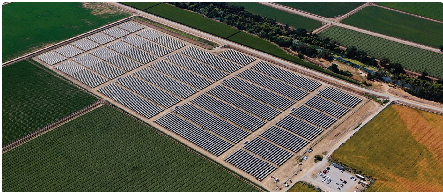
Solar farm at the University of California, Davis.
