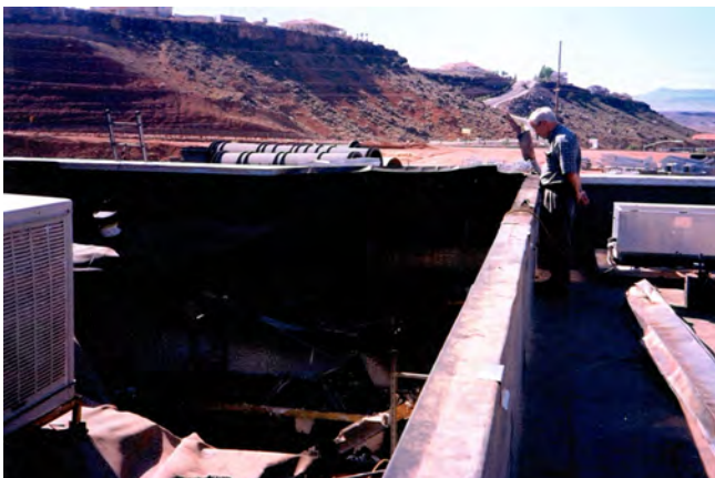
Cannery director Dale Hicken looks over damage caused by a roof fire at the cannery on April 29, 2003.
