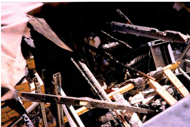
The cannery is filled with debris following a fire on April 29, 2003.
