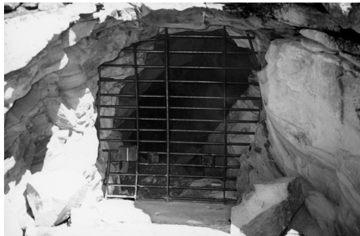
Figure 19. Typical adit grate installation designed to keep people out and let bats come and go. A removable bar permits authorized people to enter the mine for bat censuses or mineral exploration.
